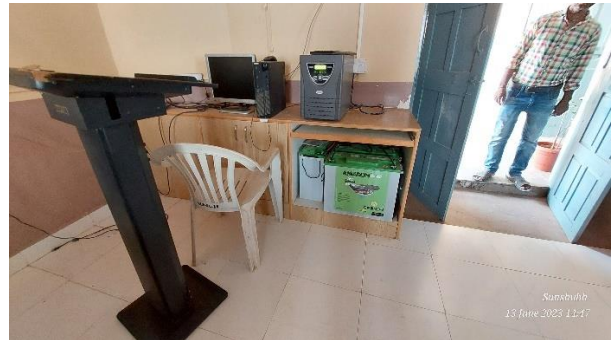
Batteries stacked without ventilation.
