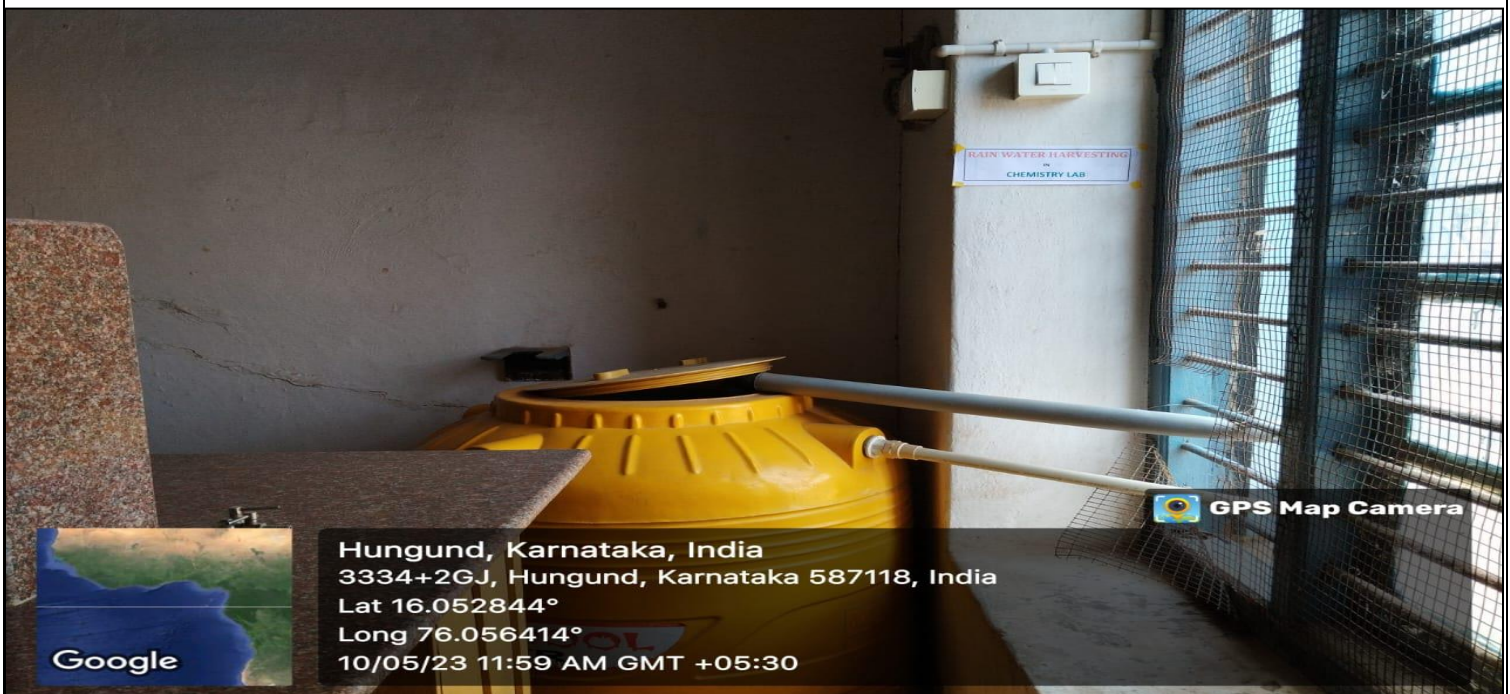
Rain water storage in chemistry lab
