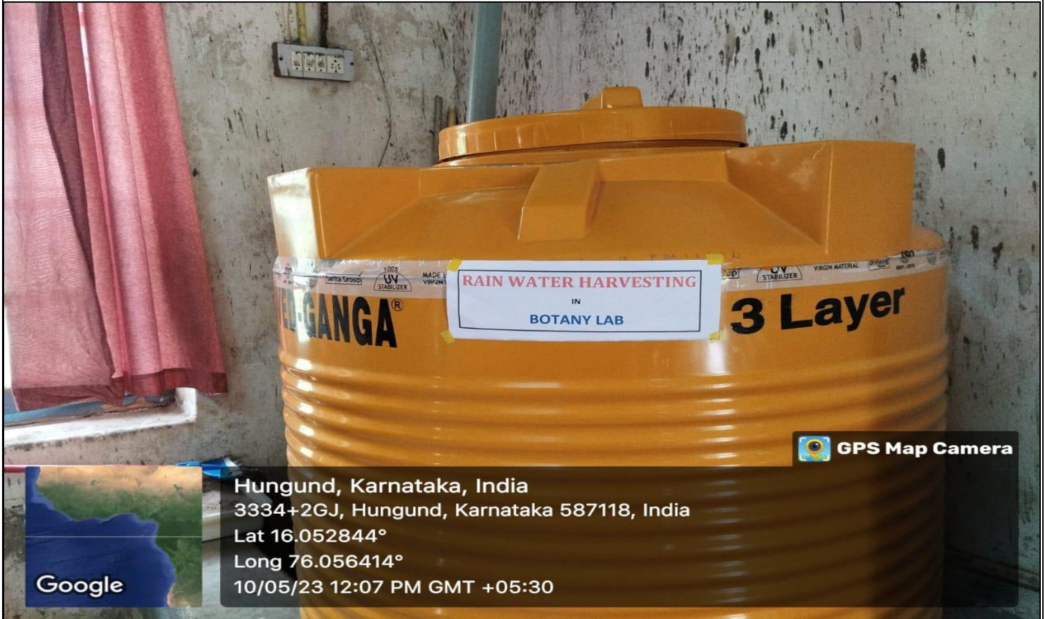
Rain water storage in botany lab
