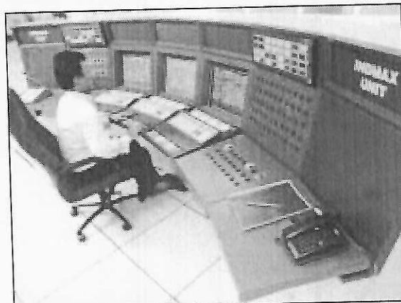
Control panel for IndMax unit at IndianOil's Guwahati Refinery - a proprietary technology for maximising LPG yield.
